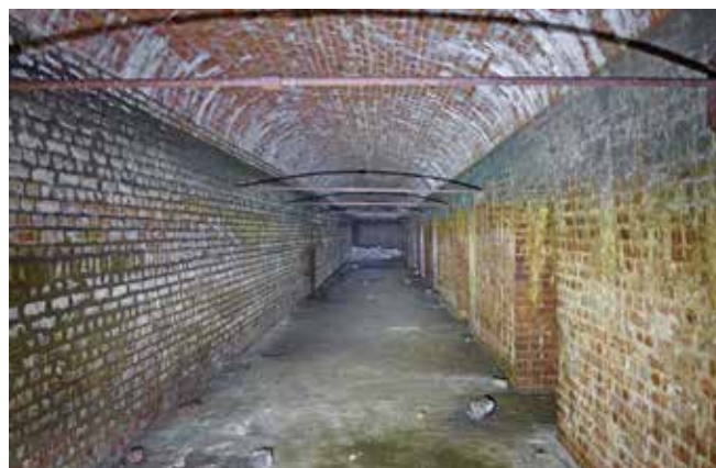
Grantham Reservoir: part of the length of the furthest chamber; note the repointed side wall
